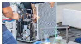
HVAC, Air Conditioning & Services
