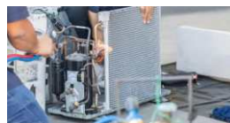
HVAC, Air Conditioning & Services
